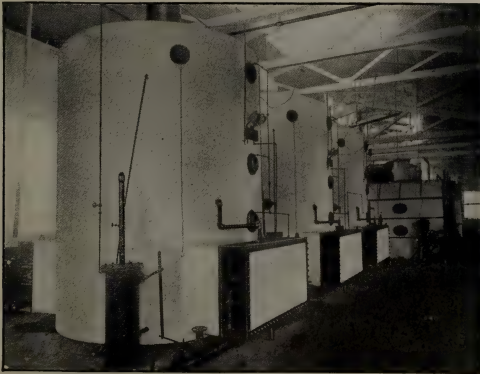
A 5000 gallon per hour Triple Effect installed for West Virginia Pulp and Paper Co., Tyrone, Pa.
